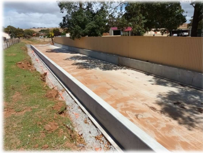
Bruce St Eudunda Drainage
